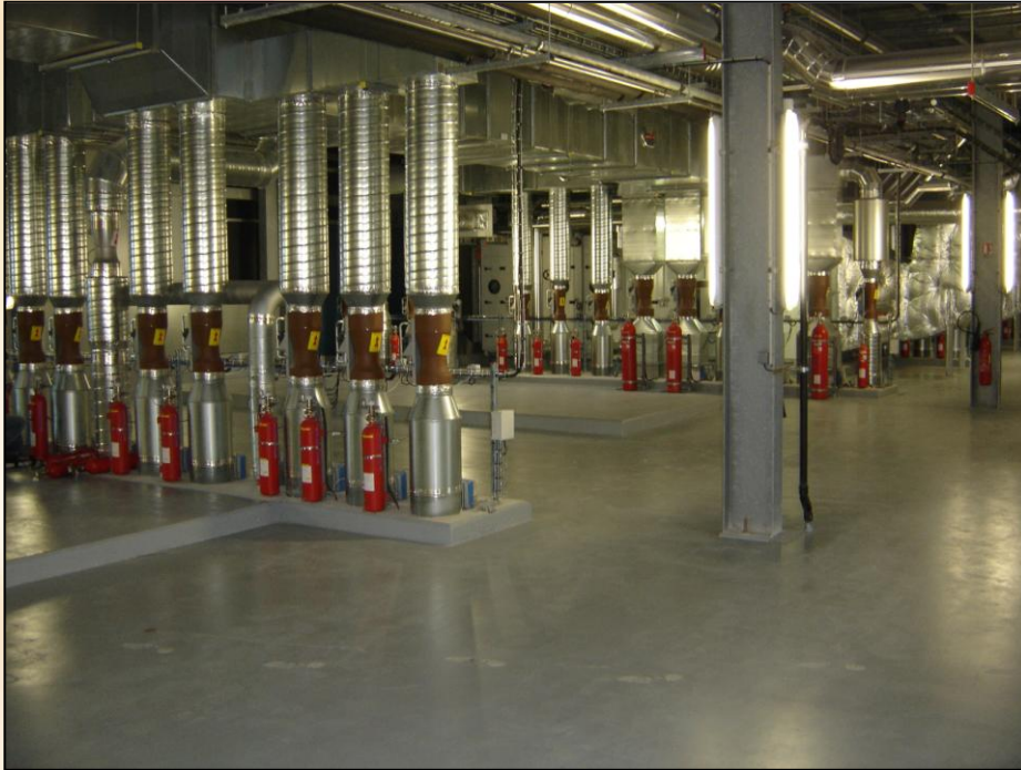
Above shows CO 2 systems used to protect the extractions system for a large pharmaceutical company
